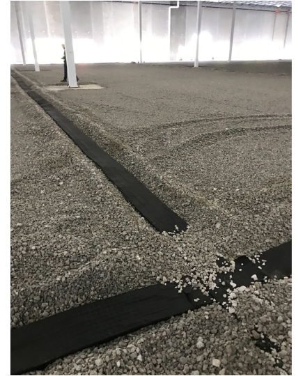
TerraVent installed flush with subgrade
